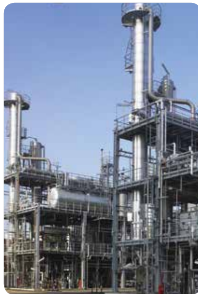
Chemical processing plants
