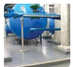
Plant Rooms and Maintenance
